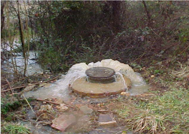
This is an actual sanitary sewer overflow caused by an oil and grease blockage.
