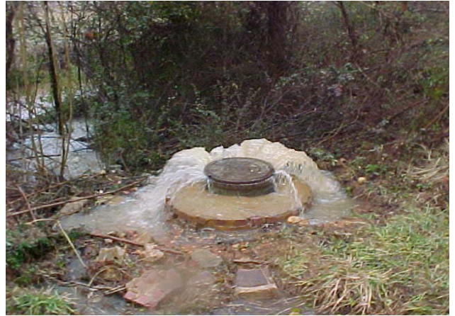
This is an actual sanitary sewer overflow caused by an oil and grease blockage.
